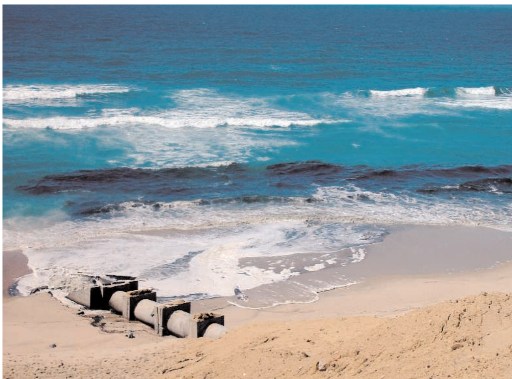
Danger signs. Sewage gushes out onto Gaza’s beaches from a failing wastewater treatment plant. Plans to upgrade the infrastructure remain frozen.
