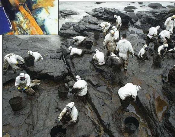
Damage control. A robotic arm patches a gushing leak on the Prestige (top) as workers last month scoop up muck from a rocky beach in northwestern Spain.
